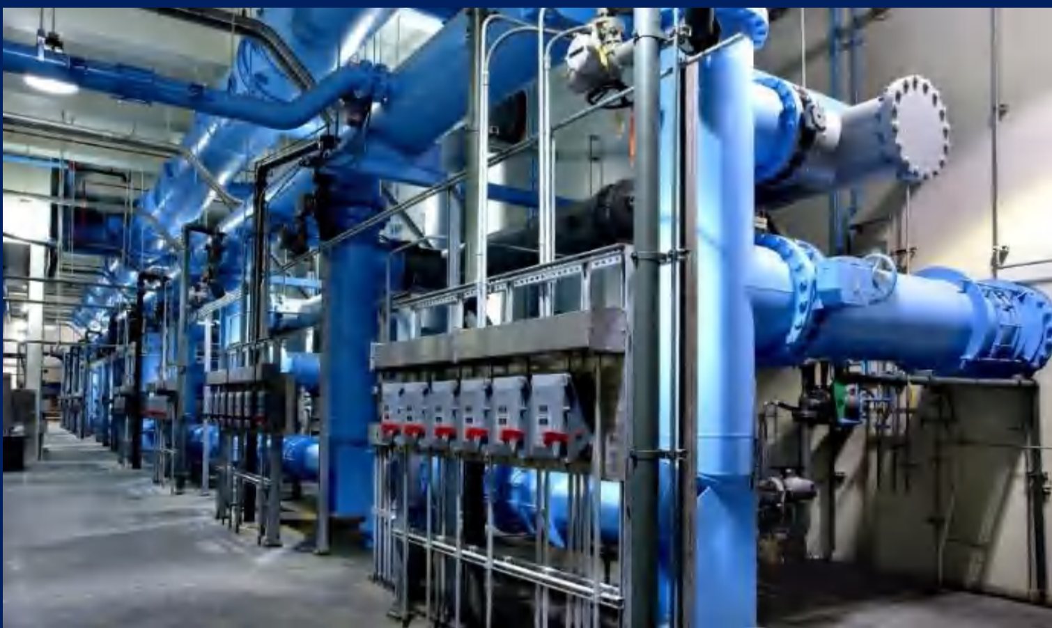
WATER PURIFICATION PLANTS
