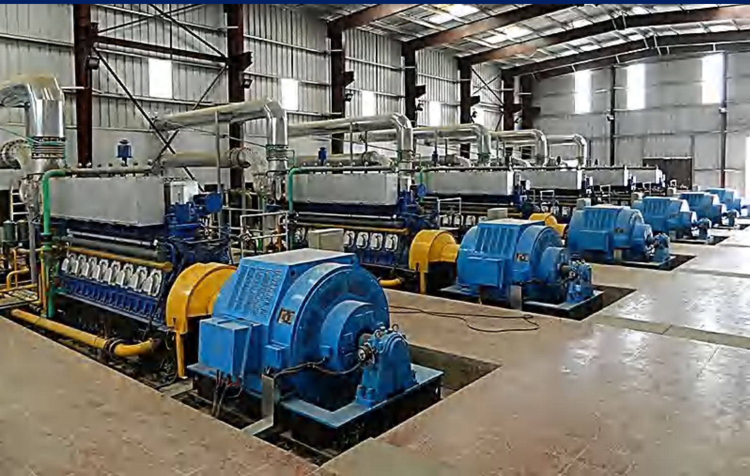
ELECTRIC POWER PLANTS (DIESEL, FUEL OIL, GAS)
