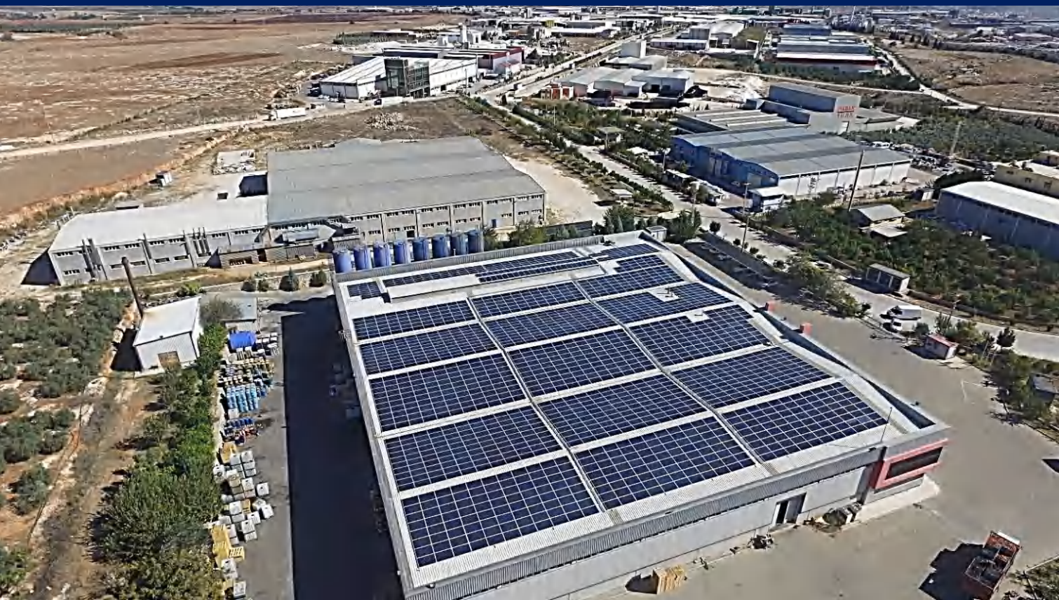
SOLAR POWER PLANTS (ROOF-TOP OR ON-THE-GROUND)
