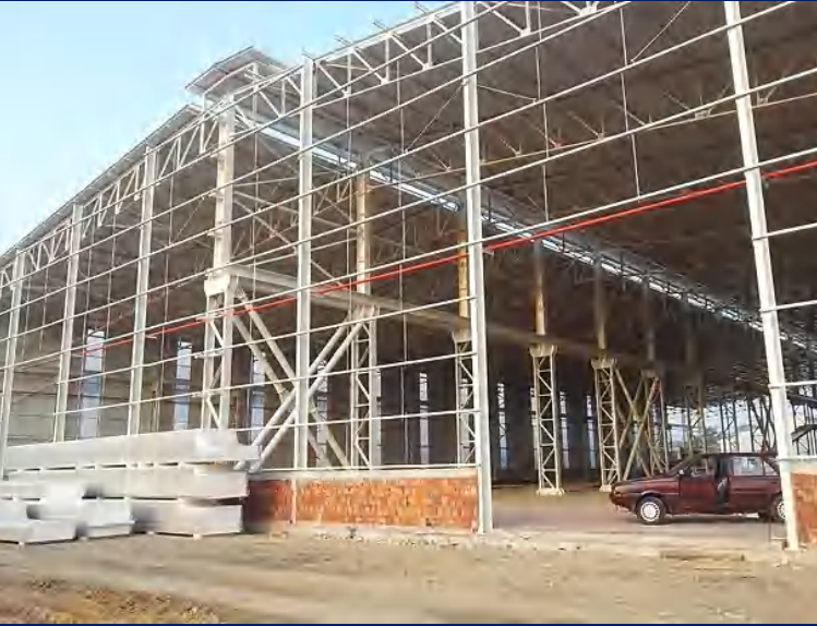
HEKIM YAPI FACTORY BUILDING-SAKARYA
